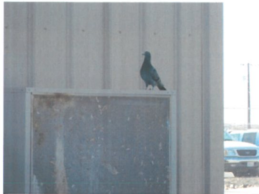
AOA Building Used as Pigeon Roost
